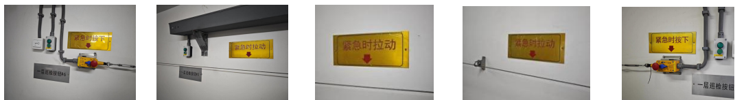
辐照室内拉线开关
