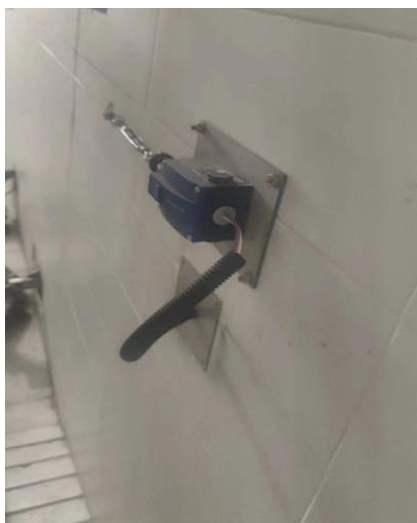
5#机房辐照室拉线开关
