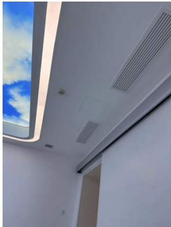
(a) SPECT/CT检查室排风
