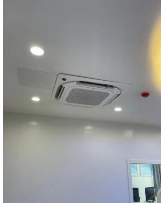
(a) PET/CT检查室排风
