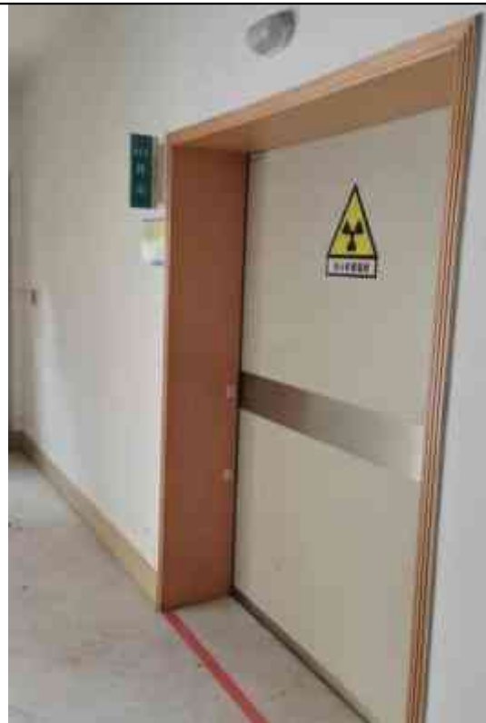
(b) SPECT/CT机房防护门
