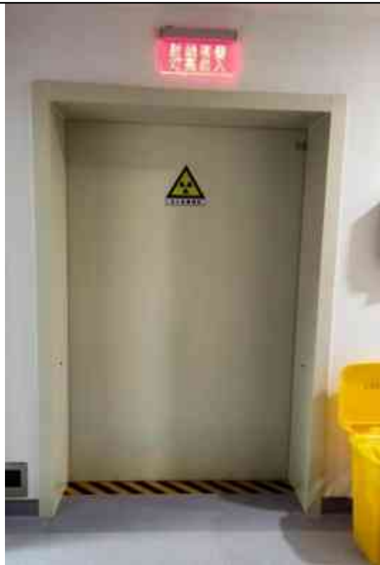
(a) DSA机房防护门
