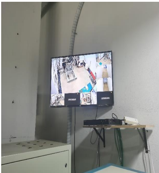
监控系统显示屏
