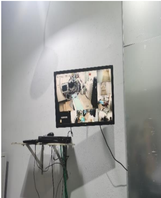
监控系统显示屏
