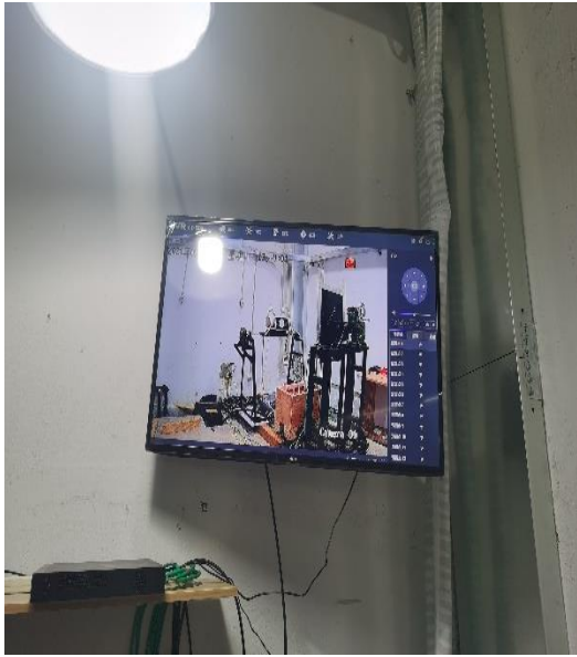
监控系统显示屏
