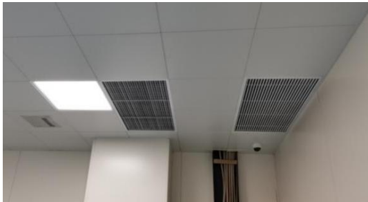
(c) SPECT/CT机房排风
