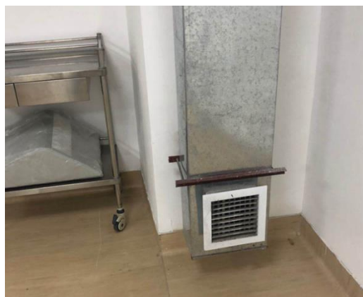
SPECT/CT 机房排风
